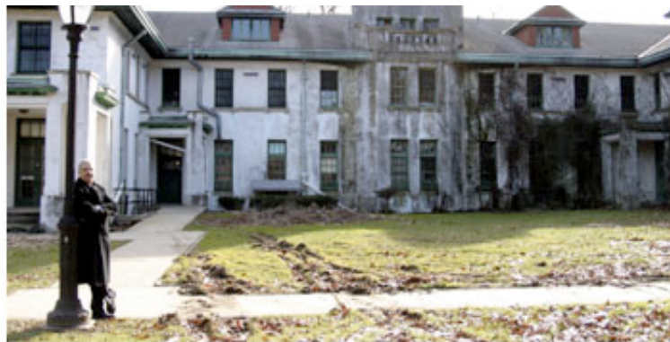
Sea View COO Tom Matteo in front of the Nurses' Quarters, which will be renovated and converted into 100 units of senior-citizen housing by 2006.
